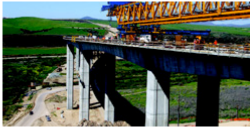
The typical spans between columns of the South Bay Expressway's Otay River Bridge measure 300 feet, or about the length of a football field. Photo: South Bay Expressway
